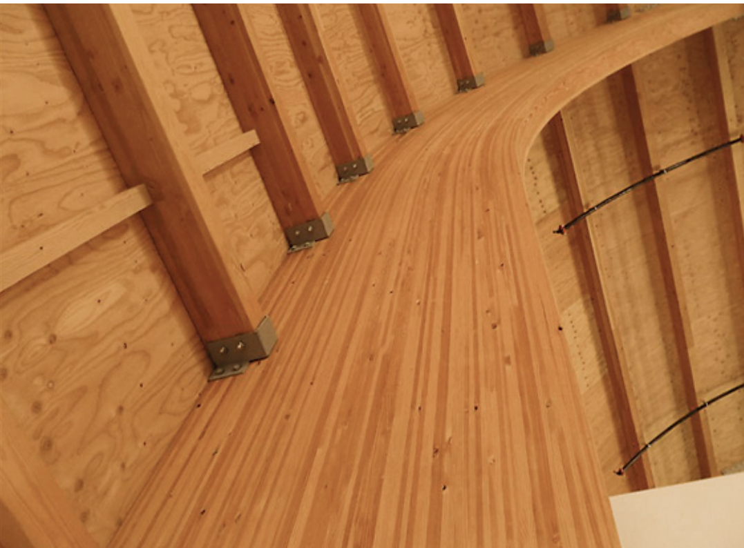
The LeMay Museum in Tacoma, Wash., features a curved roof made of custom glulam members and purlins.
