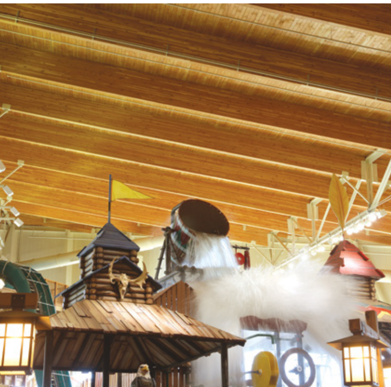
The Great Wolf Lodge in Grand Mound, Wash., features 65-foot glulam beams over the enclosed water park.
