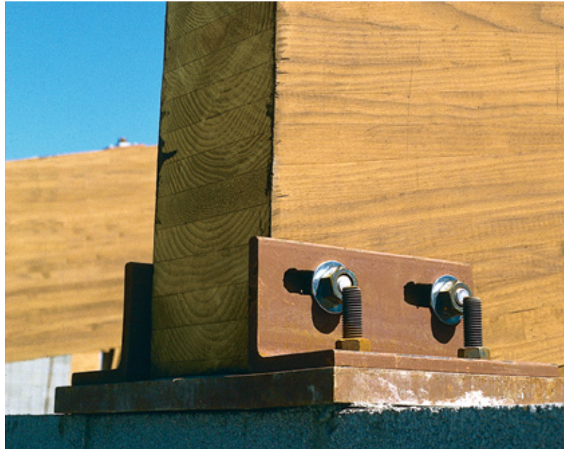
Slotted bolt holes permit horizontal movement of pitched and curved glulam beam.
