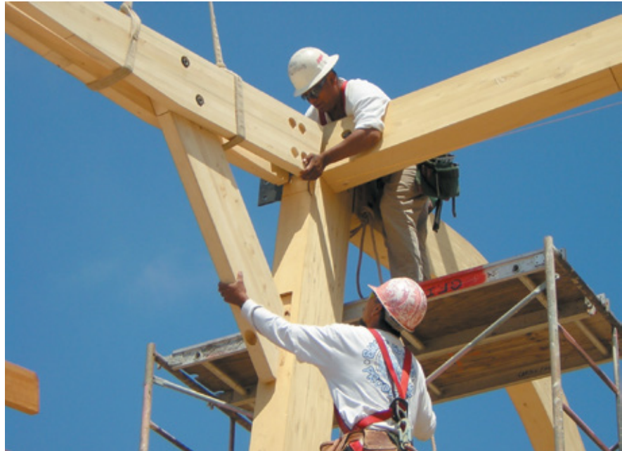
Holes and notches must be precisely located and detailed for architectural appearance and accounted for in the design of beam connections and column capacity.
