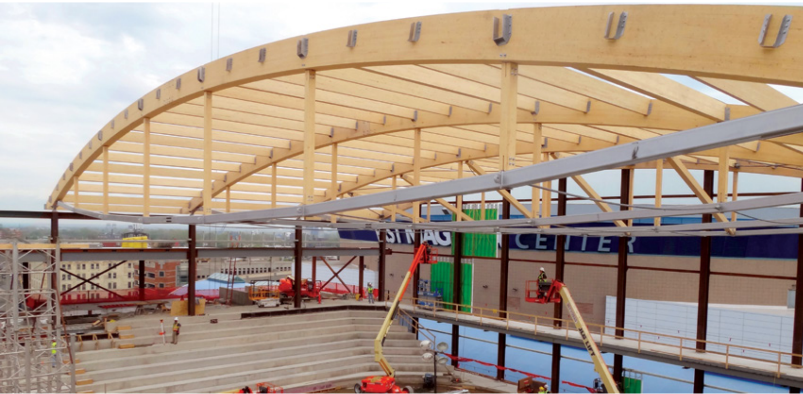
Hybrid trusses combine glulam arches, glulam purlins, and steel bottom chords at HarborCenter in Buffalo, N.Y.
