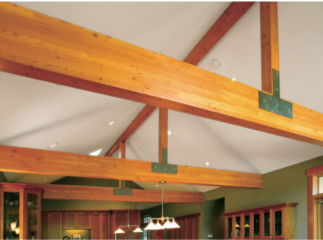
Exposed glulam ridge beams and intermediate supports for this condominium residence provide both visual drama and structural integrity.
