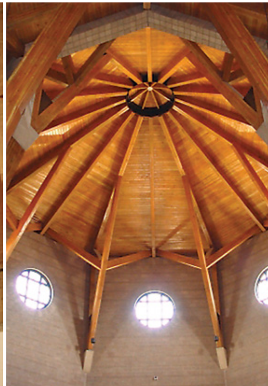
Our Lady of Loreto in Foxfield, Colo., uses three glulam members connected by a central dome.
